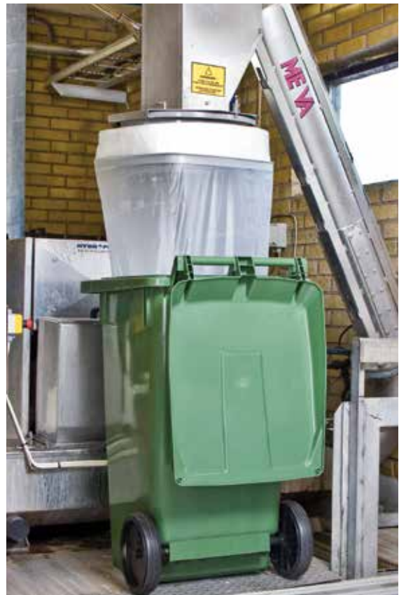
Staffanstorp Municipal Sewage Treatment Plant in Sweden has installed a Longopac Fill for the handling of screenings.
